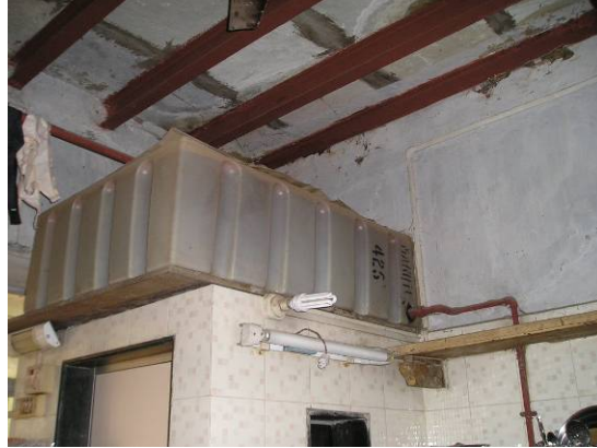
Fig.25: 500 liter water tank installed above mori , chawl at Naigaon.
