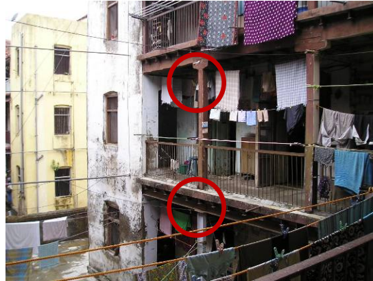
Fig.30: Steel W-sections and timber posts supporting corridors, case study 1 chawl at Naigaon.
