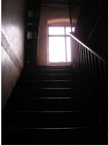
Fig.34: Sagging Treads of the timber staircase, chawl at Naigaon. Source of Image: Taken by Author
